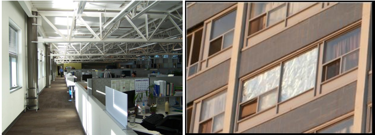
Figure 1: A shield was mounted to the top of a cubical wall to protect the adjacent occupant from a beam of light that penetrated through a gap in the shading system (left); a sheet of foil was used to cover a window to either block light or solar radiation (right).
