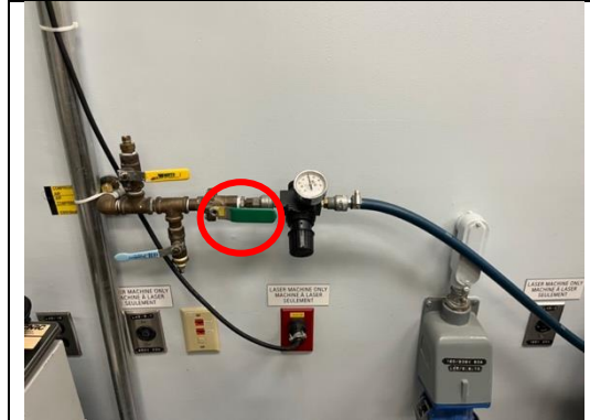
Compressed air Valve on Back wall
