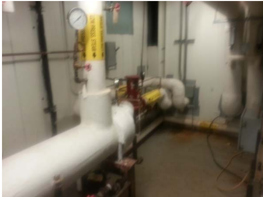
Steam to Hydronic Heat Exchanger
