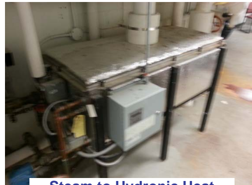
Steam to Hydronic Heat Exchanger
