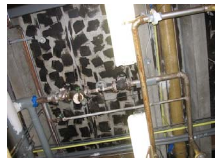
Un-insulated Steam Piping
