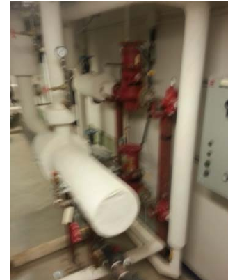
Steam to Glycol Heat
