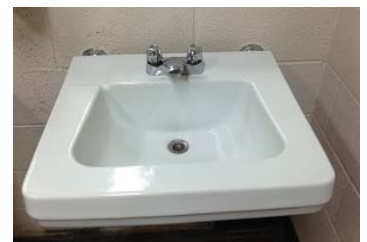
Washroom sink with low flow
