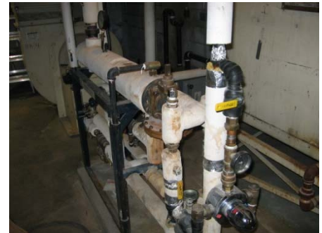
DHW Heat Exchanger
