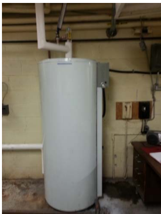
Electric Heater Tank
