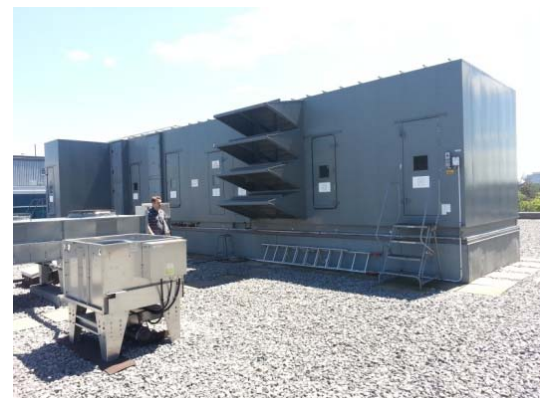
AHU-1. Serves Entire
