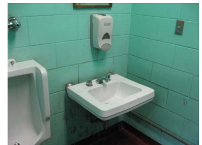
Typical Washroom Sink
