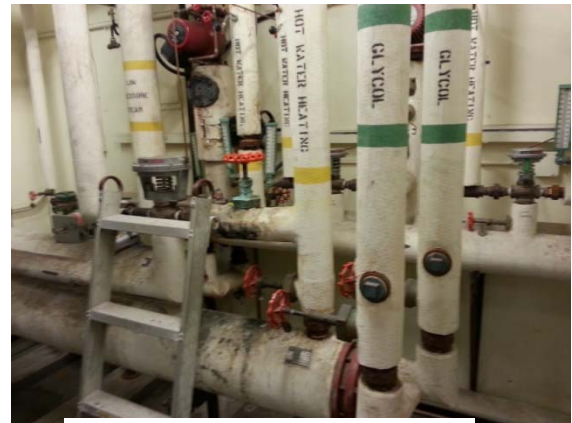
Steam to Glycol Heat
