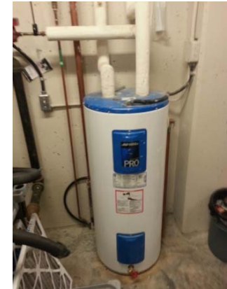
Electric Heater Tank, Newer, In Good Operating Condition
