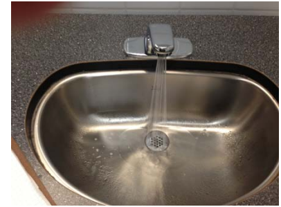
Washroom sink with ultra low flow aerator
