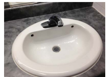
Washroom sink with low flow
