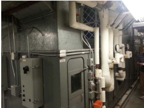
AHU-1 equipped with glycol heat reclaim loop
