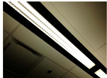
32W T8 Lighting on O/S
