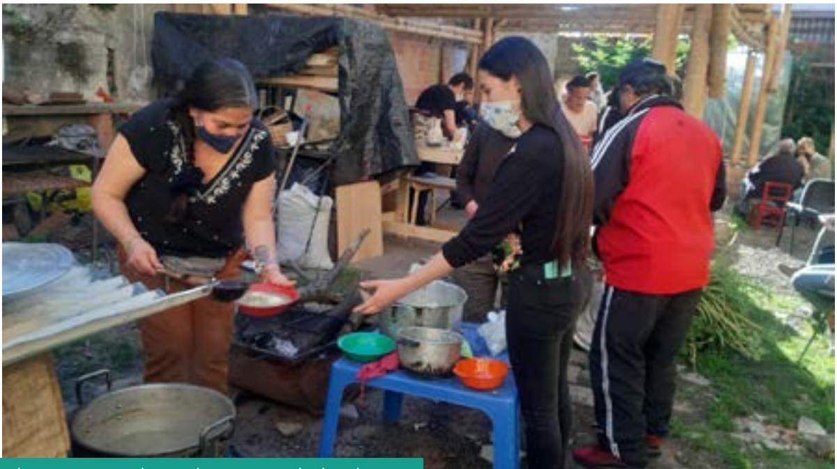
Team ID80 and community members in the community kitchen they are constructing in the neighbourhood of Bélen in Bogotá, Colombia.
