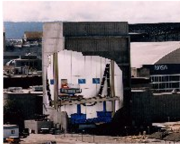
Figure 5: The NASE-AMES VMS facility.
