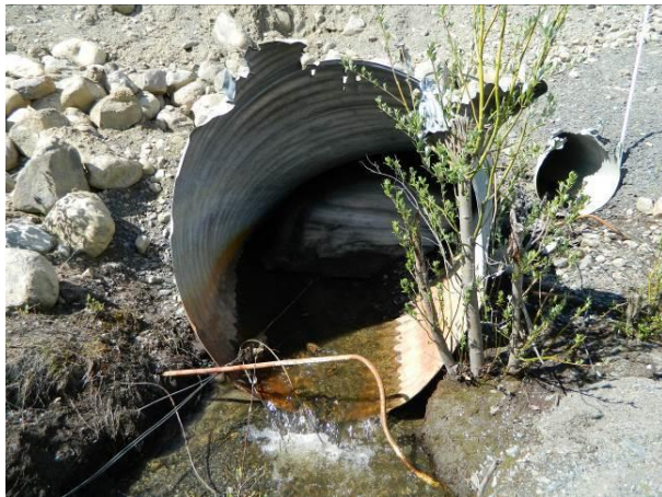
Figure 7. Culvert at km 32.5 (North Klondike River valley), filled with icing, May 2014. Photo by C.R. Burn.
