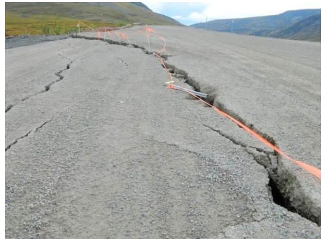
Figure 11. Thaw subsidence of the embankment at NT km 27, August 2011. Photo by C.R. Burn.
