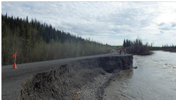
Figure 10. Wash out of the road by Ogilvie River at km 245, June 2013. Photo by S.N. Orban
