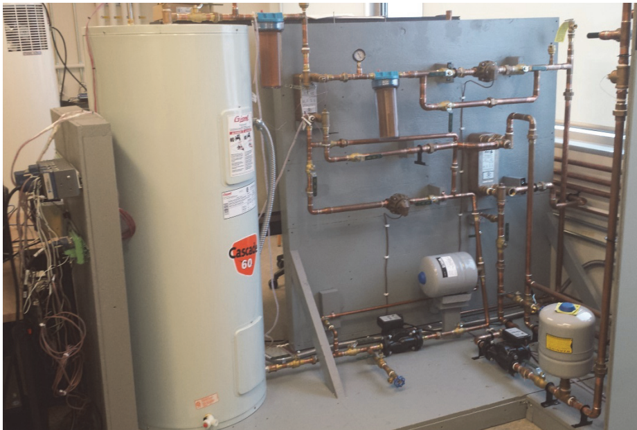
Figure 3-12:Hydraulic network installed within the lab
