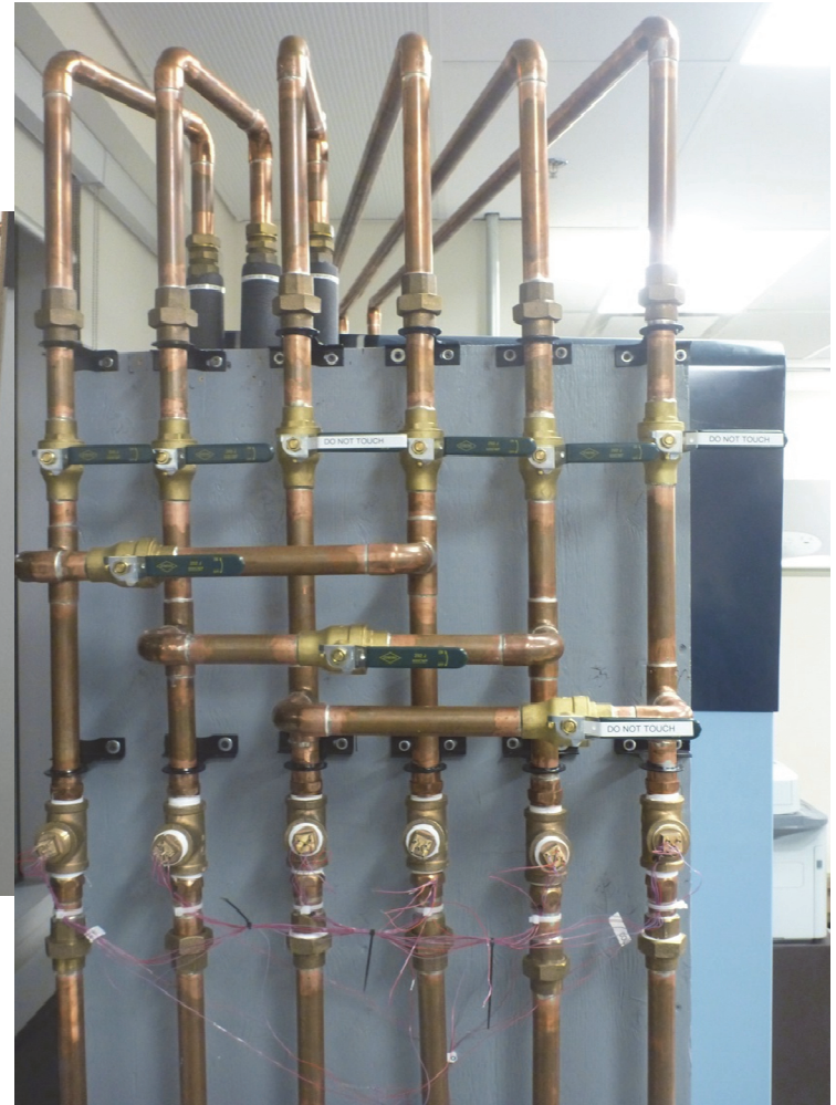
Figure 3-13: Connections into the chiller and thermopile installation
