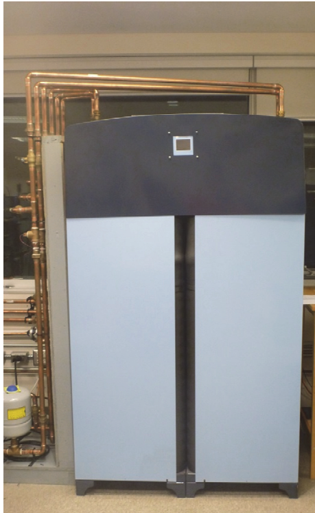
Figure 3-3: ClimateWell solar absorption chiller installed within the lab
