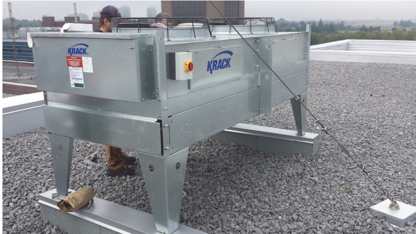
Figure 3-2: Installed dry cooler
