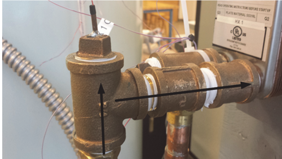
Figure 3-5: Thermowell at the entrance of a heat exchanger with the flow direction indicated
