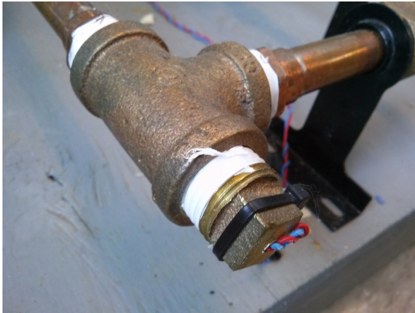
Figure 3-9: Pipe Tee Fitted with Thermocouple Probe on the HPWH Tank Drain Line
