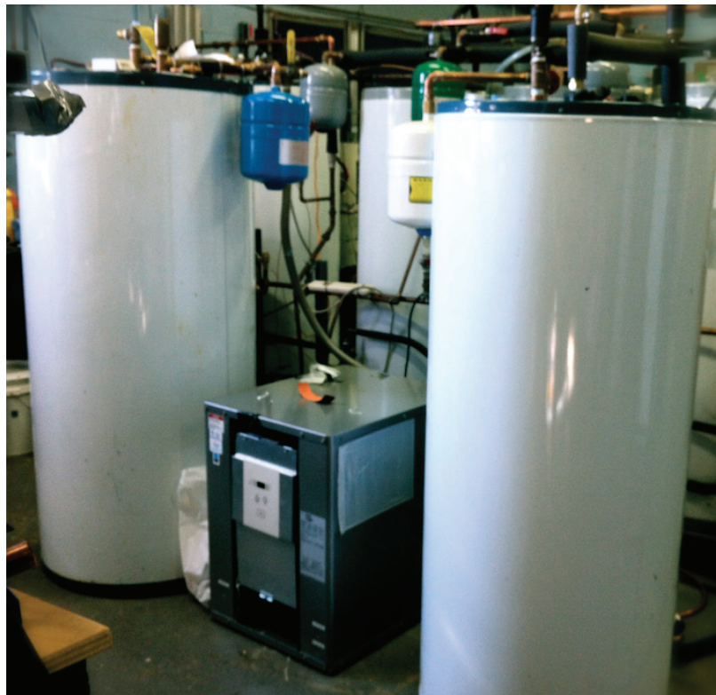
Figure 4.1: Experimental apparatus of dual tank indirect solar-assisted heat pump system
