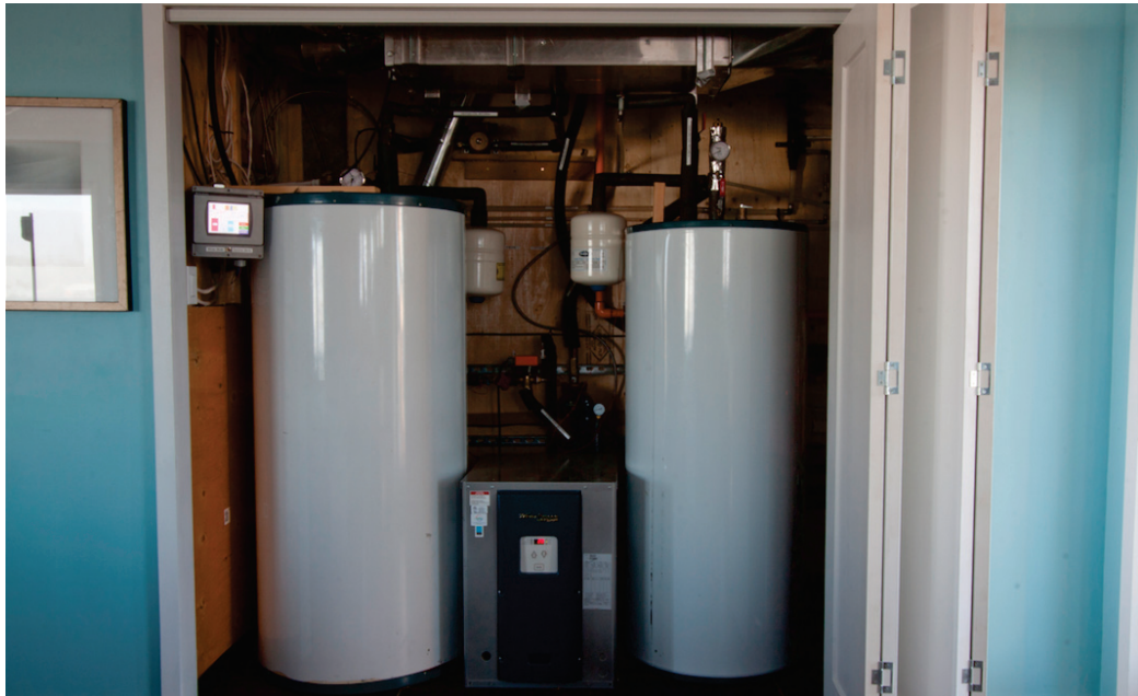
Figure 1.11: ECHO's mechanical closet containing the designed SAHP (Photo credit: Carly Farmer)
