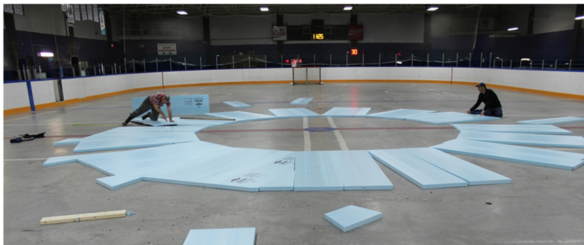
Figure 8: Layout of insulation before installation (E. Kucerak, personal photograph, April 26, 2014). Adapted with permission.
