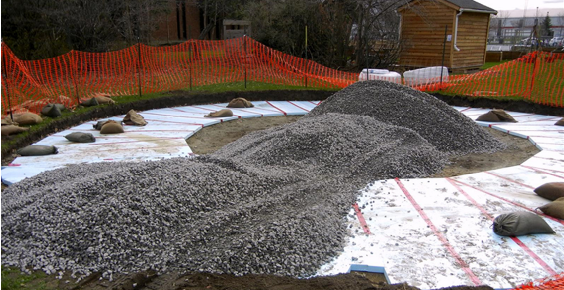
Figure 9: Installation of EPS insulation on site (E. Kucerak, personal photograph, May 2, 2014). Adapted with permission.
