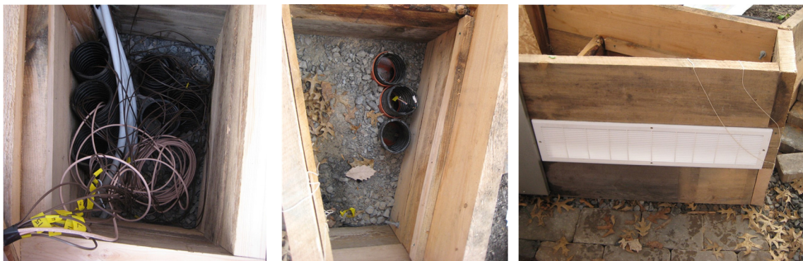
Figure 14: Earth-to-air heat exchanger air intake box (left), air outlet box 1 (middle), and air outlet box 1 vent (right).
