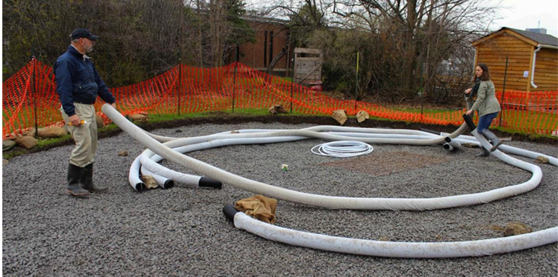
Figure 10: Layout of earth to air heat exchanger piping (E. Kucerak, personal photograph, May 3, 2014). Adapted with permission.
