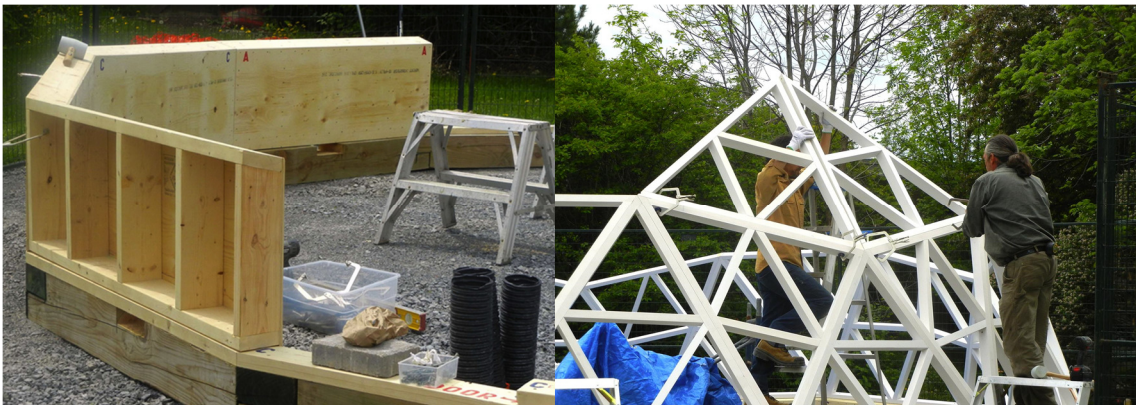
Figure 16: Installation of base walls (left) (E. Kucerak, personal photograph, May 26, 2014) and trusses (right) (E. Kucerak, personal photograph, May 29, 2014). Adapted with permission.
