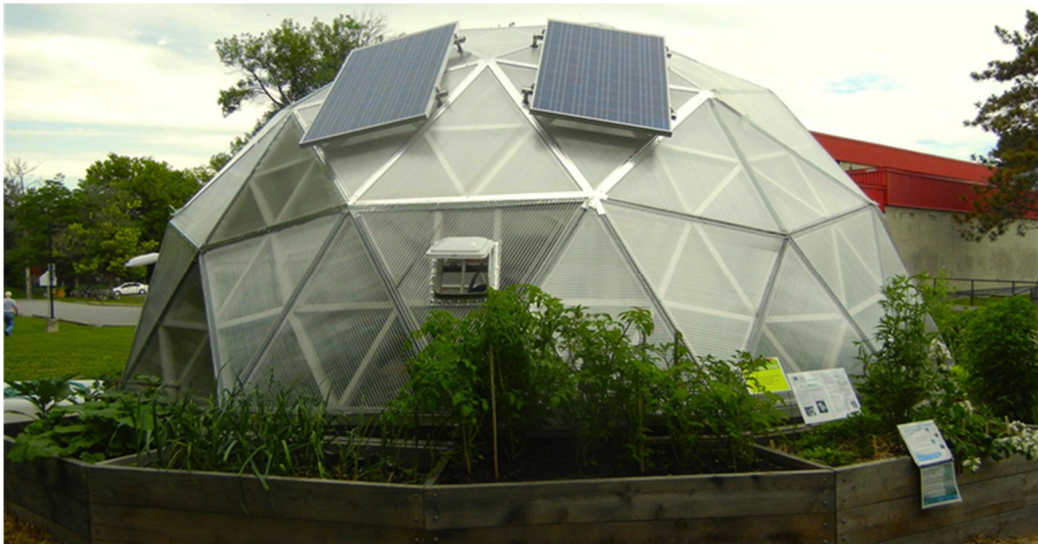
Figure 23: Installed solar panels (E. Kucerak, personal photograph, June 25, 2015). Adapted with permission.
