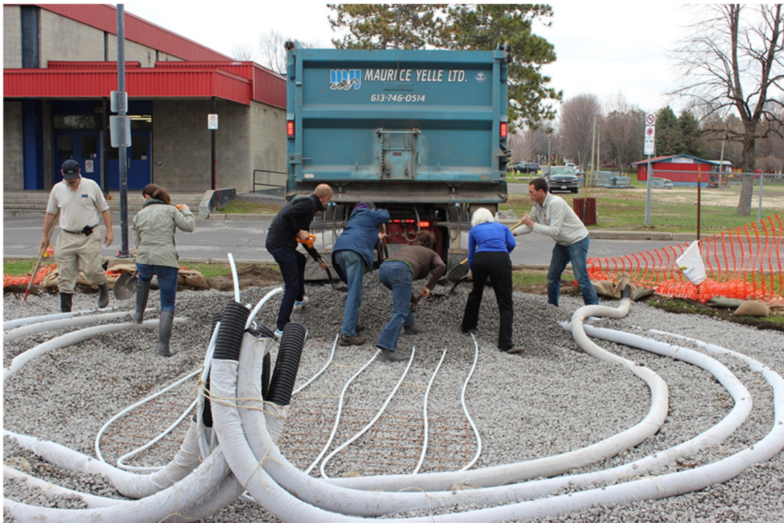
Figure 11: Installation of earth to air heat exchanger piping (E. Kucerak, personal photograph, May 3, 2014). Adapted with permission.
