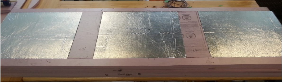
Figure 3-15: Construction of a composite panel with VIPs encased in XPS with top sheet removed
