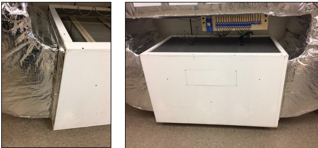
Figure A.11 Left) Ducting Tap used to Seal PCM Box to Duct and b) Completed PCM Box Installed in Air-Loop
