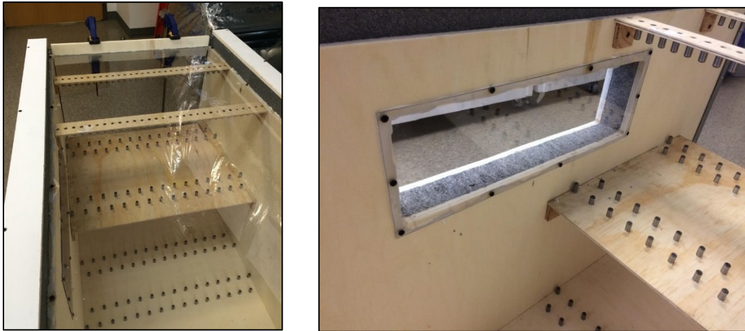
Figure A.9 Left) PCM Box with Plexiglass Installed and b) Installation of Plexiglass in Side Window
