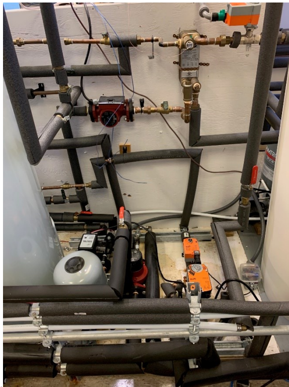
Figure 3-5: Images of the medium temperature chiller set-up, including the components of the chiller (top) and the required infrastructure to operate and test the chiller (bottom)
