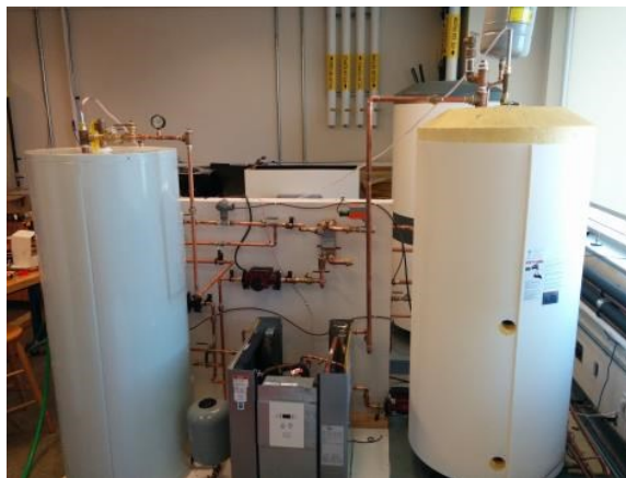
Figure 3-1: Photo of heat pump (center) with cold (left) and hot (right) thermal storage systems
